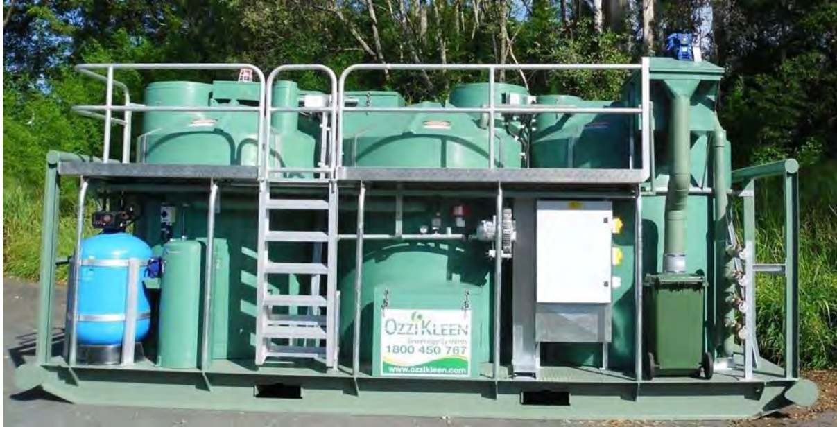
Figure 3: On-site waste treatment plant
