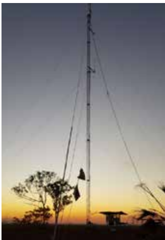
Upgraded mast has been erected and BFNT link aerial installed at Gypsy Spring
